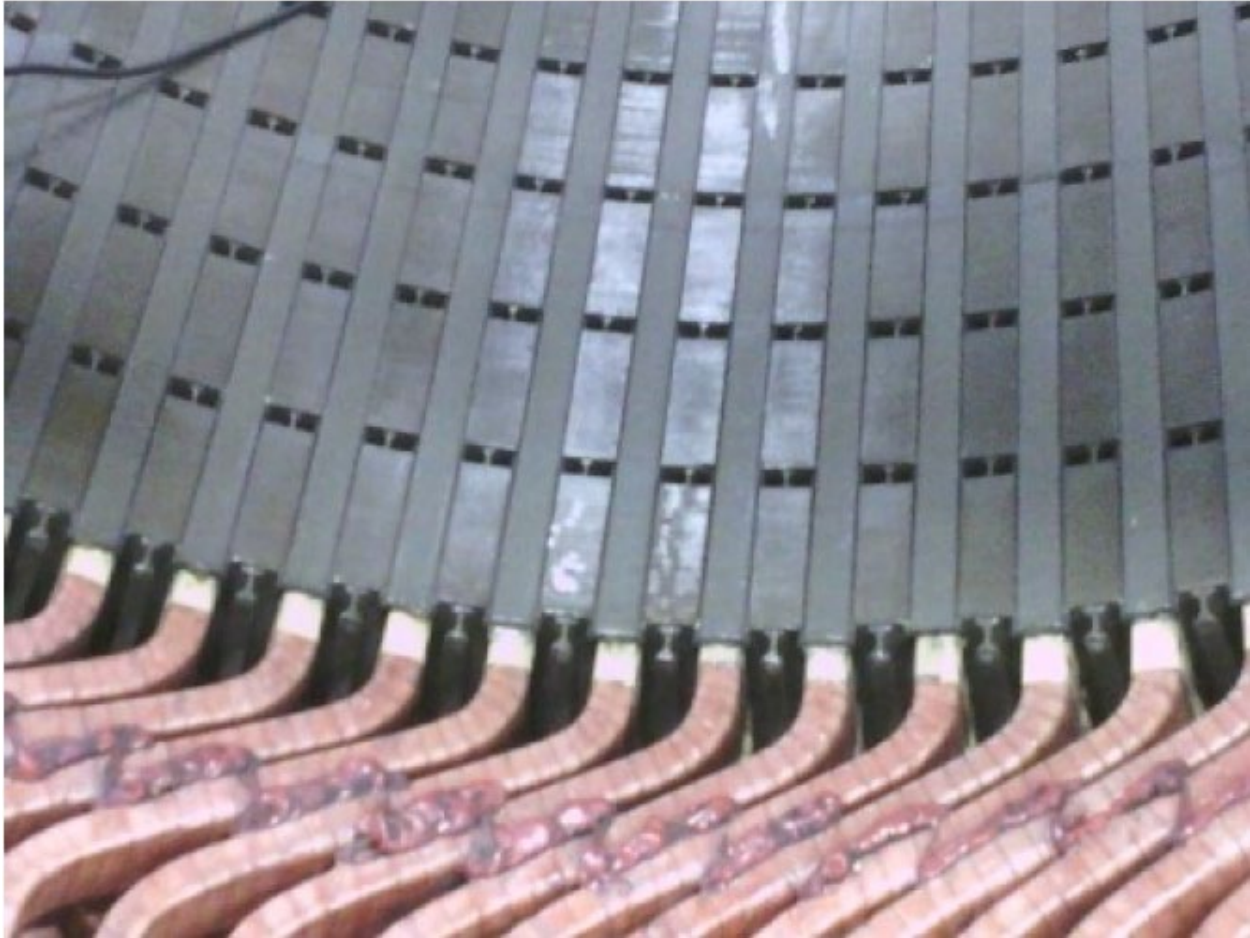
Figure 2: stator with white dots marking where hot spots were located.
