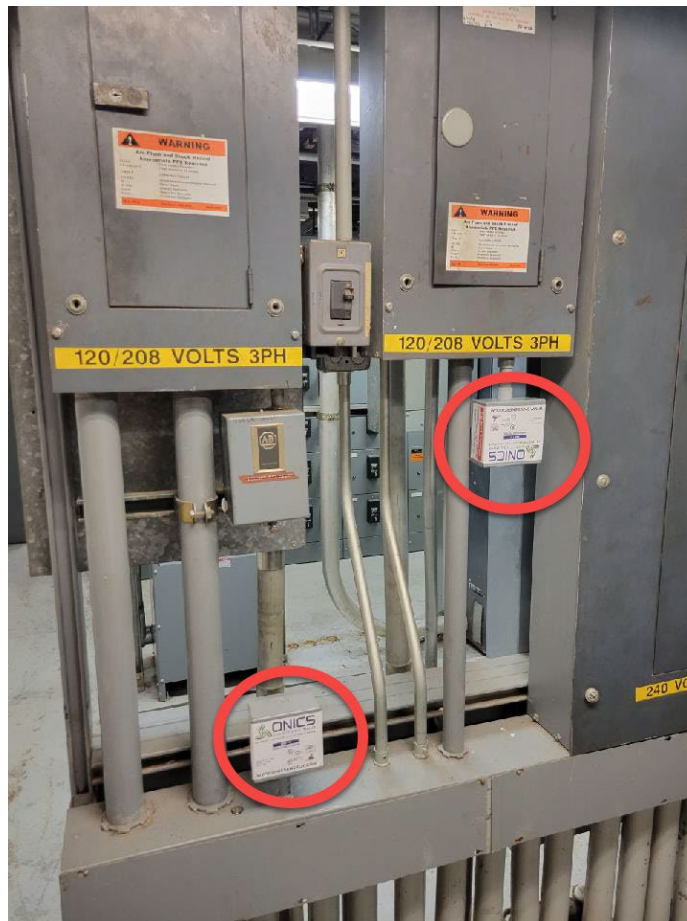
Figure 1: Onics neutral harmonics devices installed at panels.
