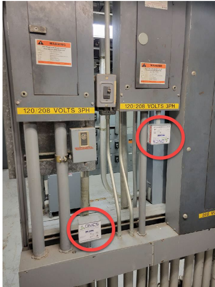
Figure 1: Onics neutral harmonics devices installed at panels.
