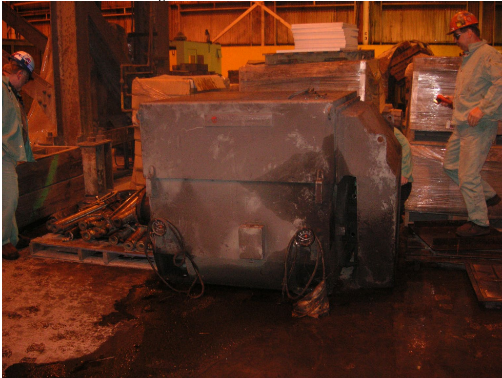
Figure 1: #4 Combustion Fan Motor
