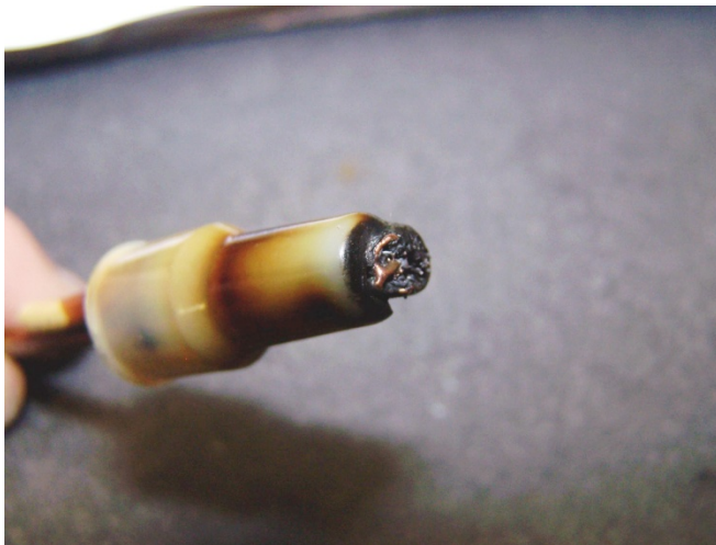
Figure 4: Defective Crimp Connection (b)
