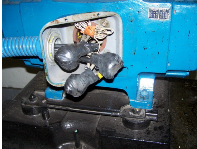
Figure 6: Too Much in the Connection Box
