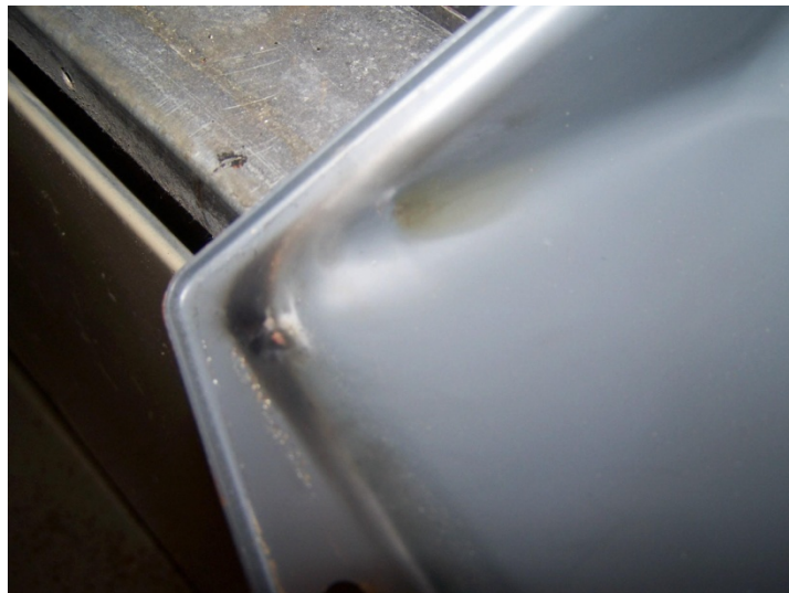
Figure 2: Connection Box Fault Point
