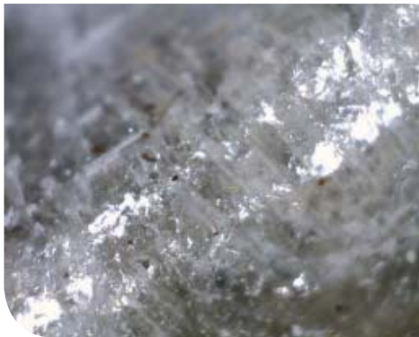
The brown material is iron dust and some other evidence of tunneling caused by what's called magnetic termites.
