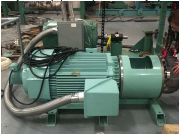
Figure 7: Pump System Setup for Full Load High Speed
