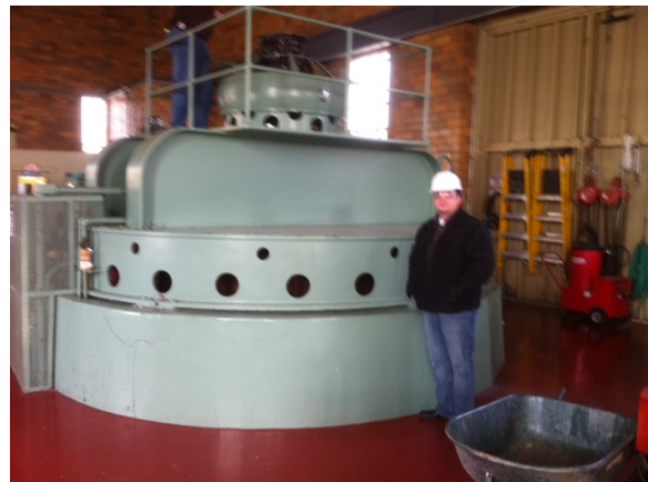
Figure 1. Generator Prior to Disassembly and Testing
