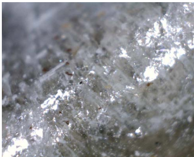
Fig. 4. Iron filings and pathways several layers deep into mica tape along top edge of top coil.
