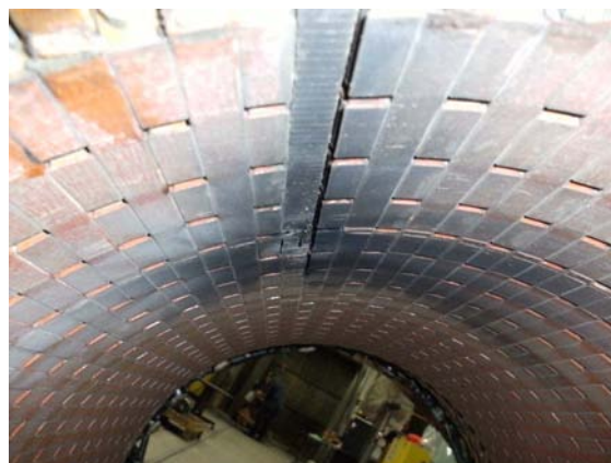
Fig. 1. Failed Stator Coil with Missing Wedge
