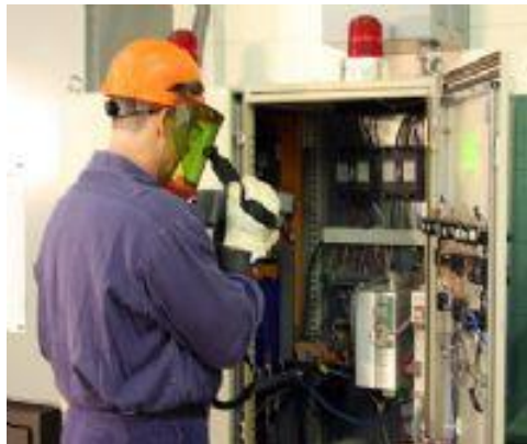
Figure 1: Infrared Thermographer Working with Open Cabinet
