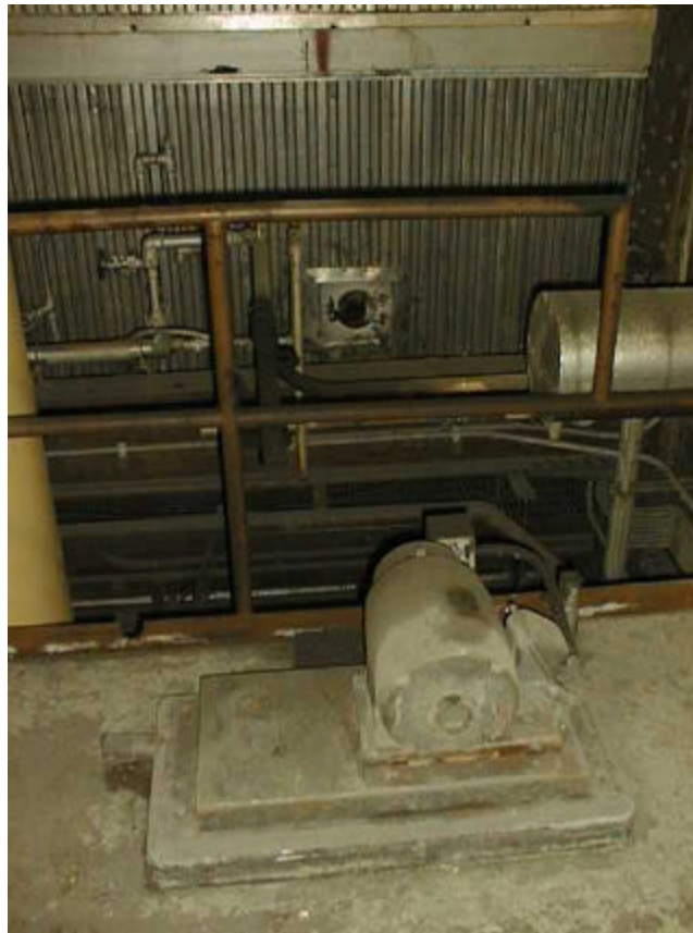
Figure: Motor No Longer In Service
