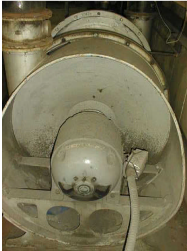
Figure 3: Bad Connection Box
