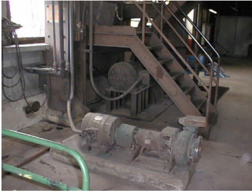
Figure: Pump No Longer In Service
