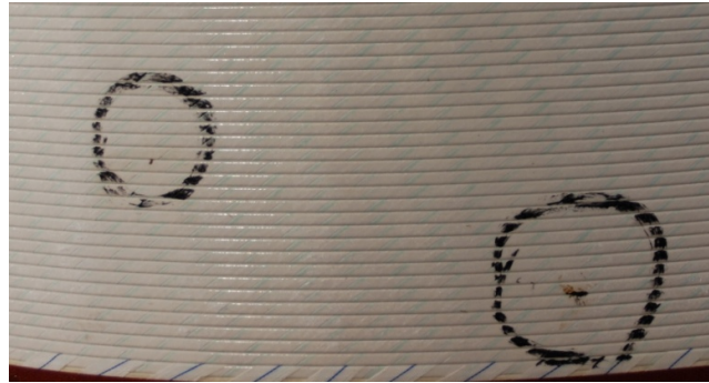
Fig 3: Burn Spots Between Primary Conductors
