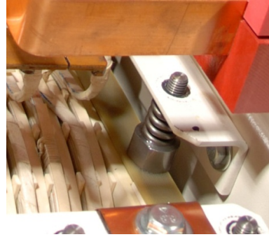
Fig 2: Fretted Bolts and Buckets
