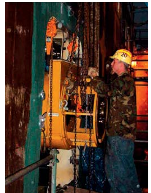
Figure 2 - Generator Removed From Mission-Critical Application Three Months After Fault Detected As Recommended
