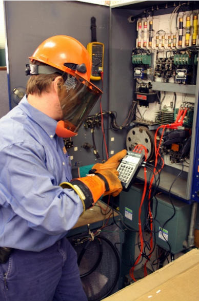
Figure 4: A technician using the ALL-TEST Pro OL ESA instrument (Courtesy: Dreisilker Electric)
