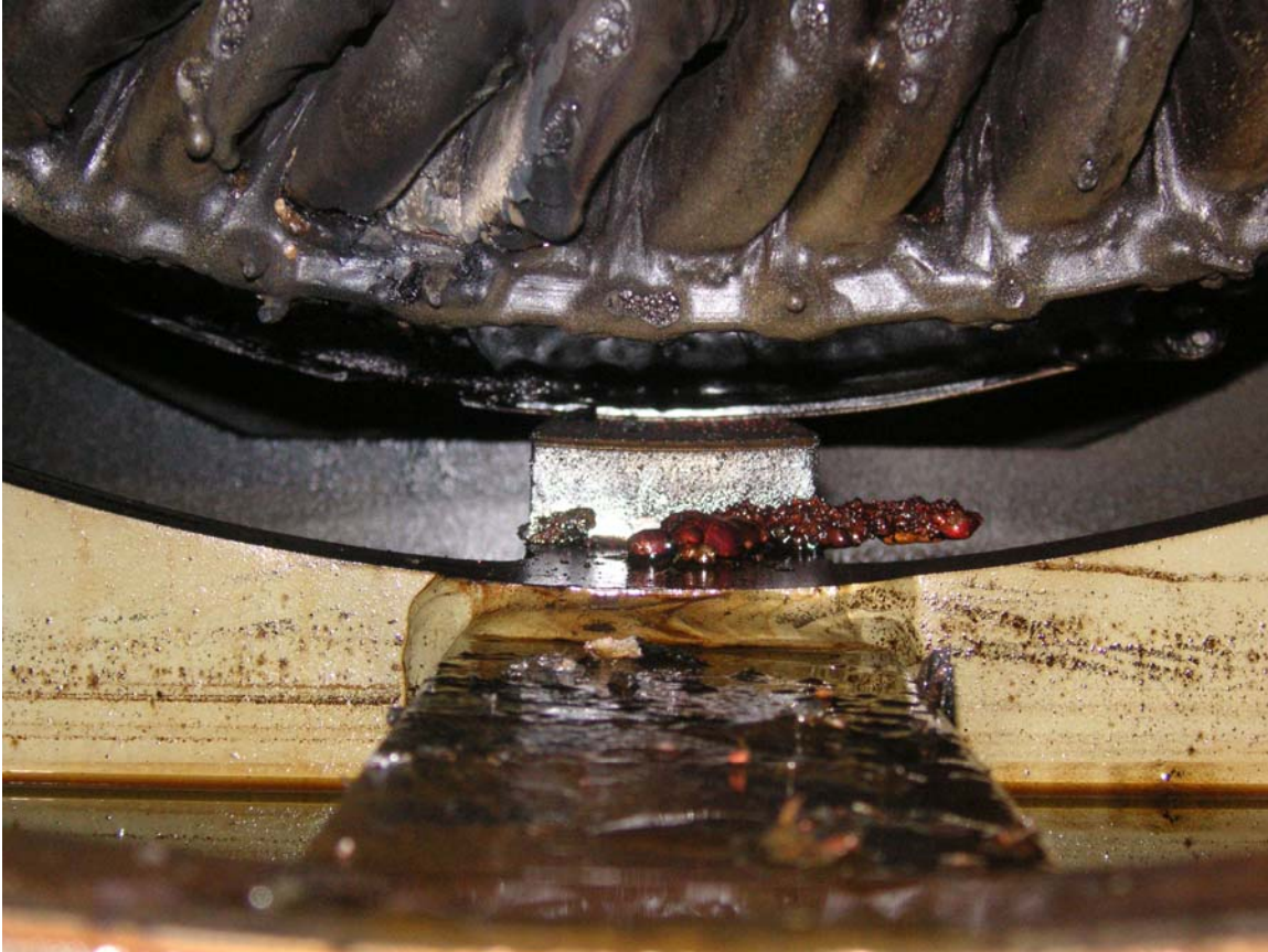
Figure 4: Copper from Louis Allis Coil Failure
