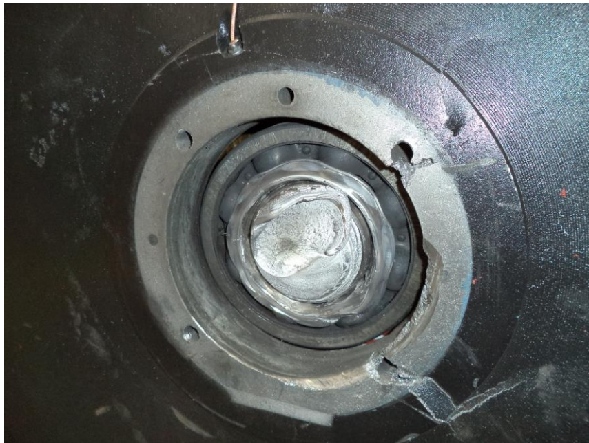
Figure 4: Broken Shaft due to Improper Tuning
